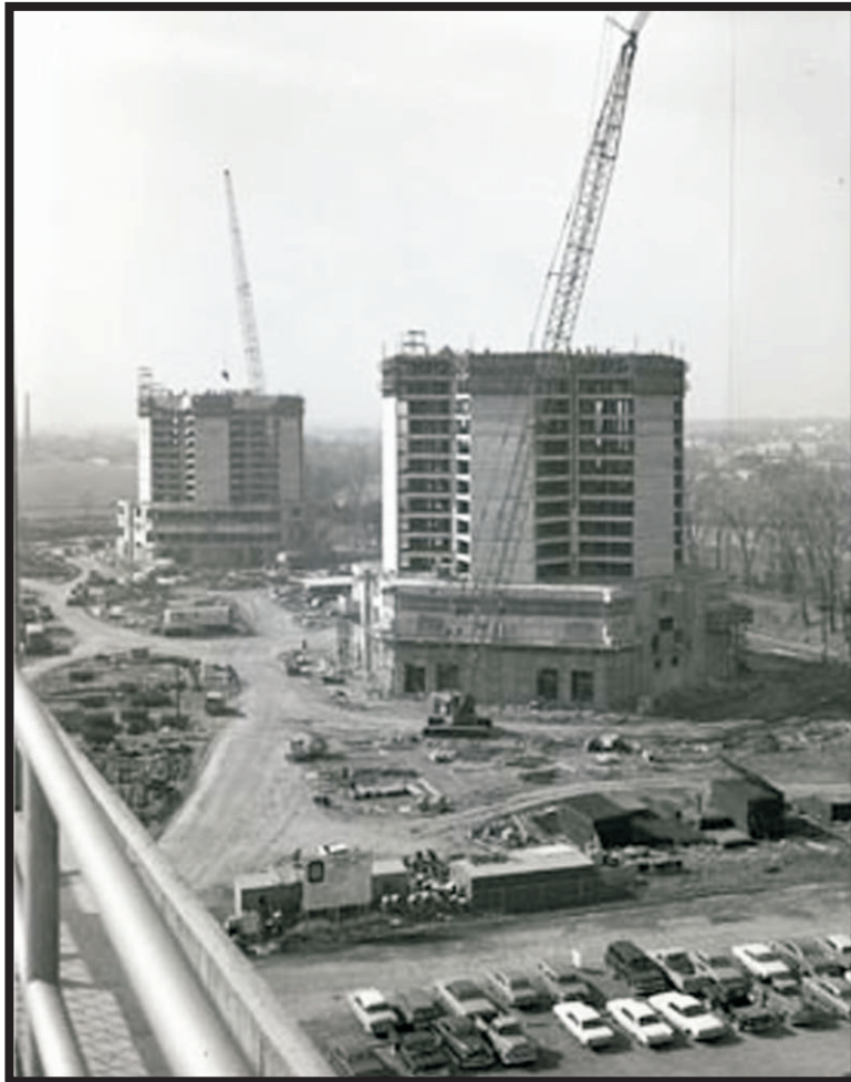
Plate B80. Morrill and Lincoln Tower construction at Ohio State University in 1966 (The Ohio State University Photo Archives 2010).
